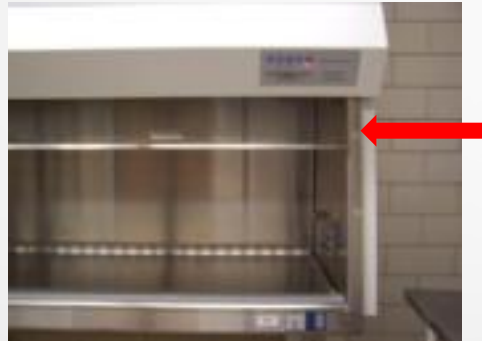
SASH TOO HIGH
